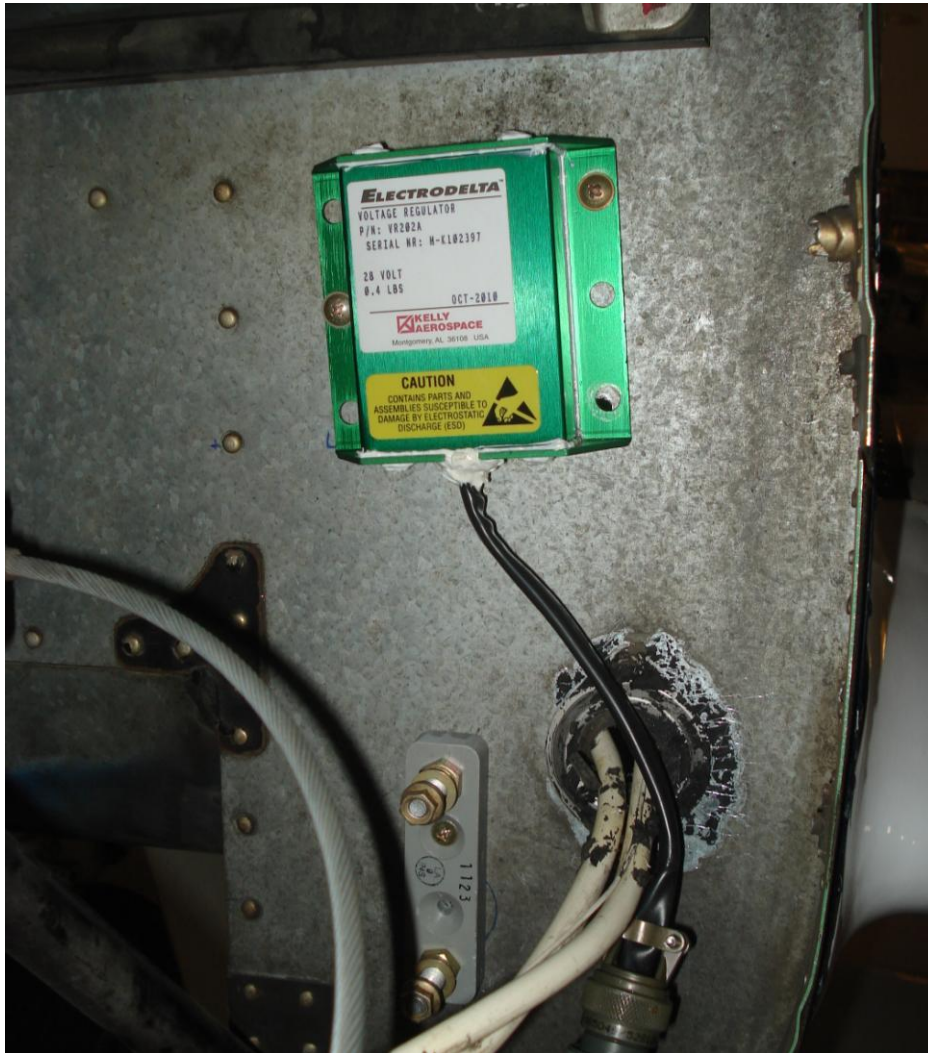
Figure 1 - Approximate location of VR-202A Voltage Regulator
