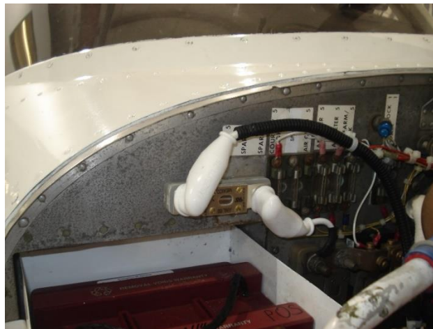
Figure 22 – Bonanza 36 Current Limiter Installation
