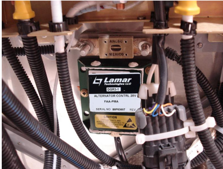
Figure 1 - Approximate location of DGR3-1 Voltage Regulator
