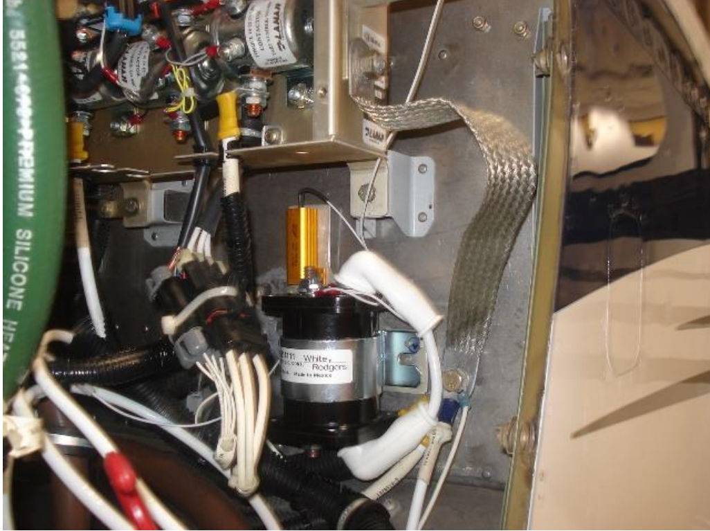
Figure 9 - Approximate location of AL-00206 Alternator Switching Relay
