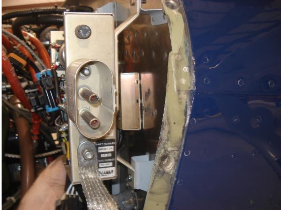
Figure 7 - Approximate location of DGR3-1 Voltage Regulator
